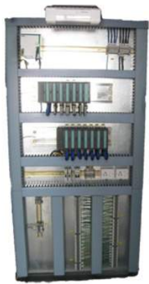
REMOTE I/O PANEL
